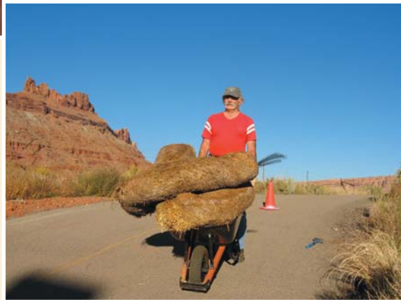
Erosion control along paved trail
